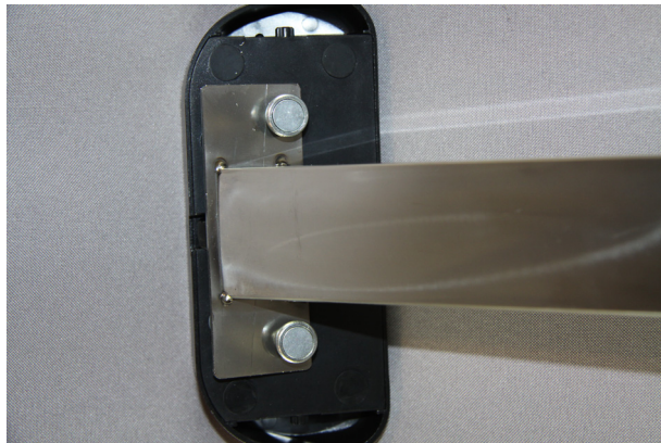
Figure 2.7 Remote Display Attached to Column
